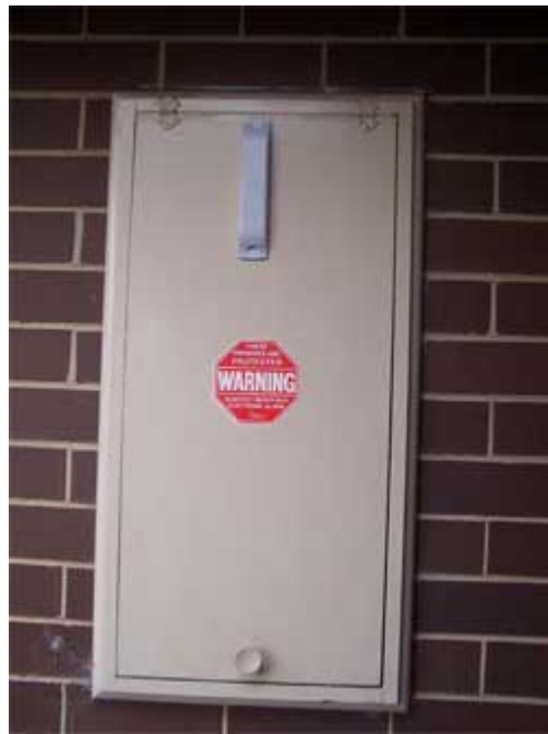
Figure 50 - SP-AUSNET Meter in Timber Box -Ext Antenna
