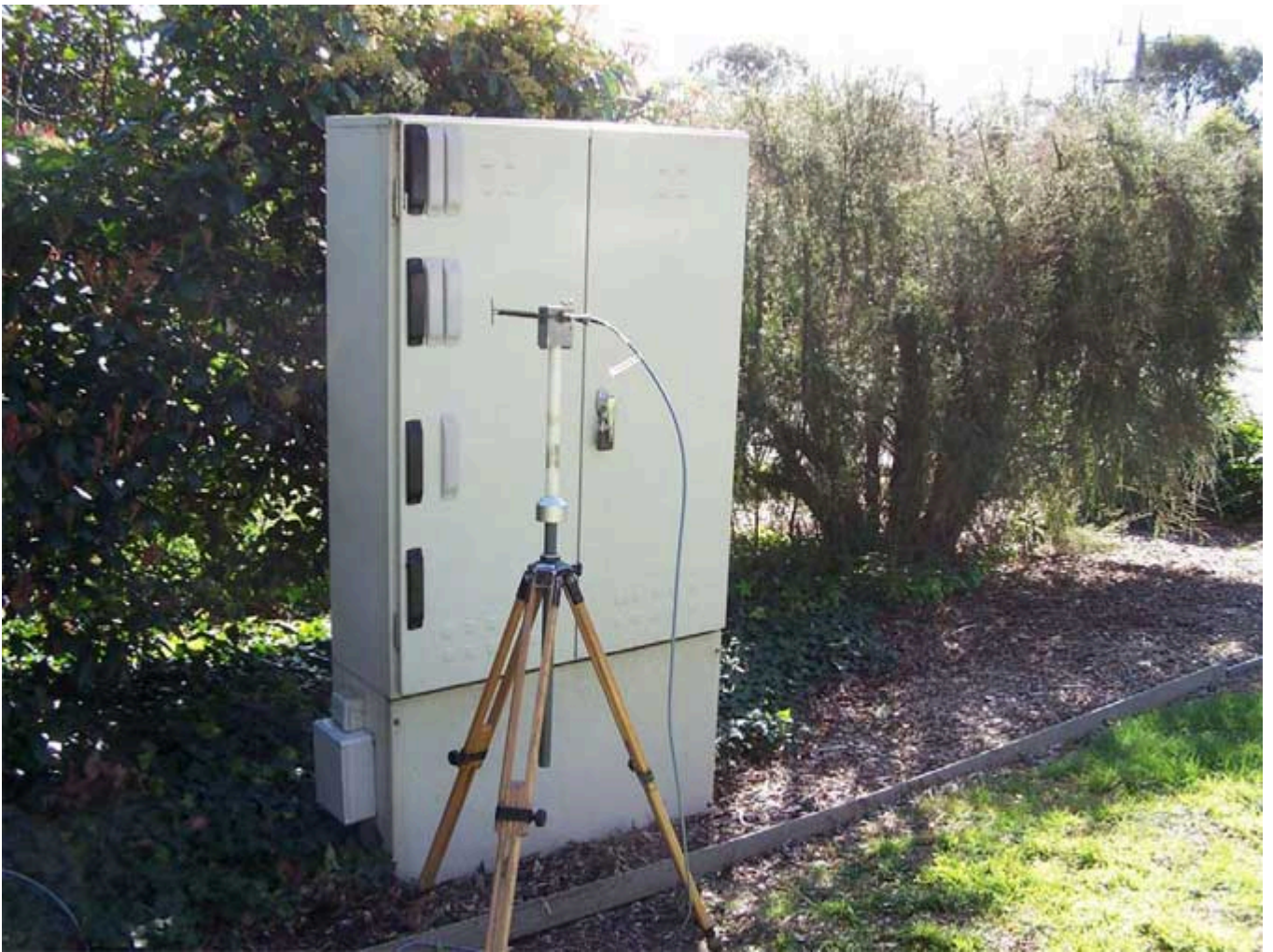
Figure 45 – SP-AUSNET Group Meter Site with External Antennas
