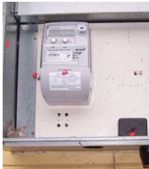
Figure 48 – Jemena Meter with External Antenna Box
