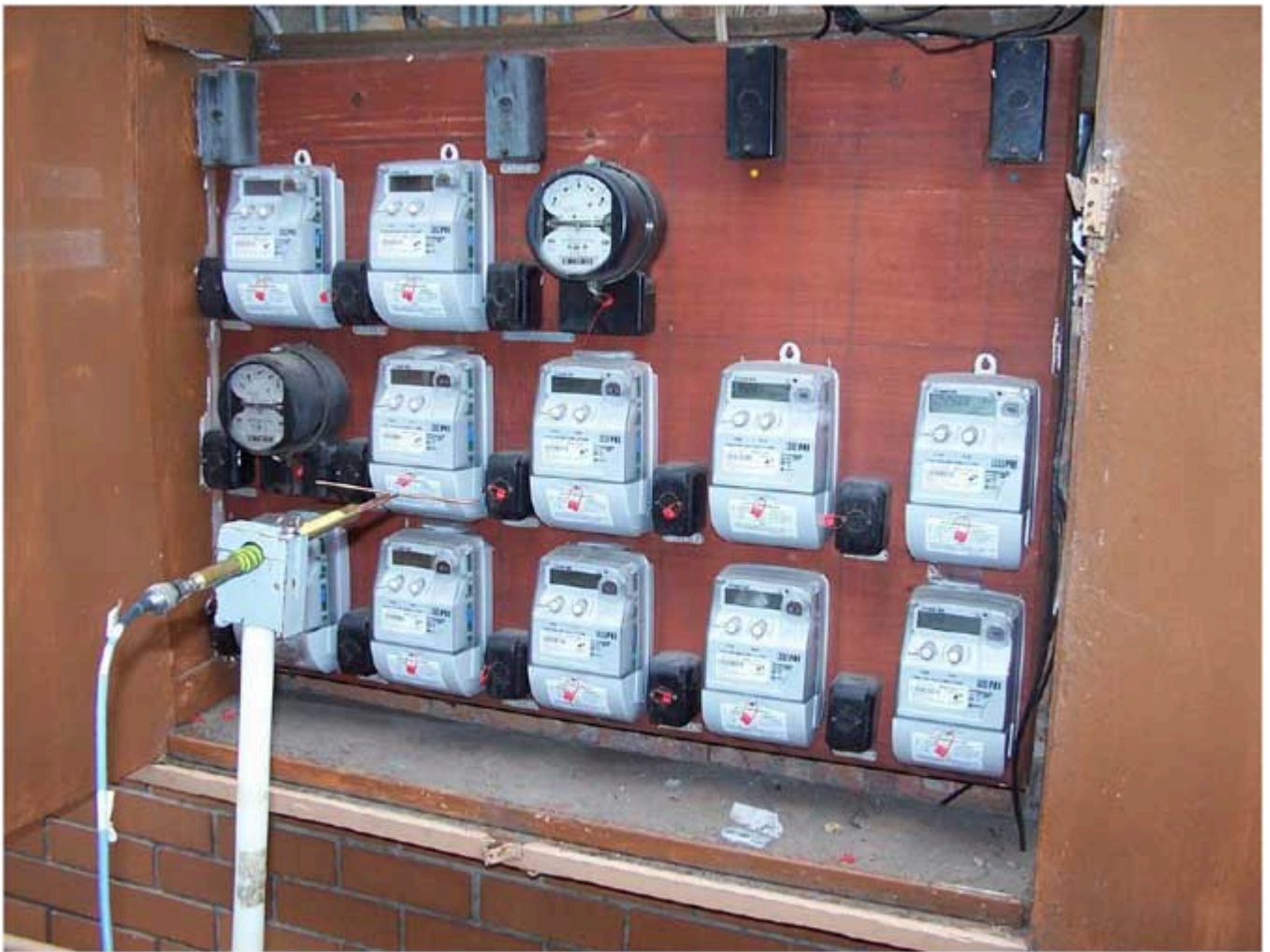
Figure 46 – Jemena Group Meter Site
