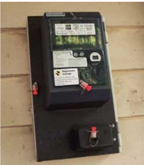
Figure 47 – Powercor Meter with no Meter Figure
