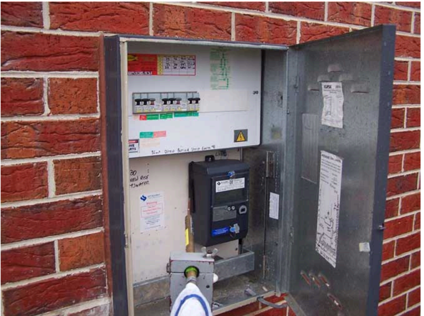
Figure 51 – SP-AUSNET Meter with Dual Antennas attached
