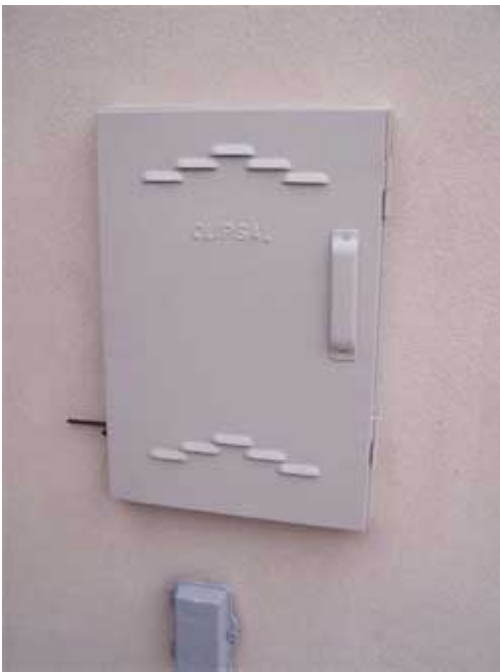
Figure 49 – SP-AUSNET Meter in Metal Box - Ext Antenna
