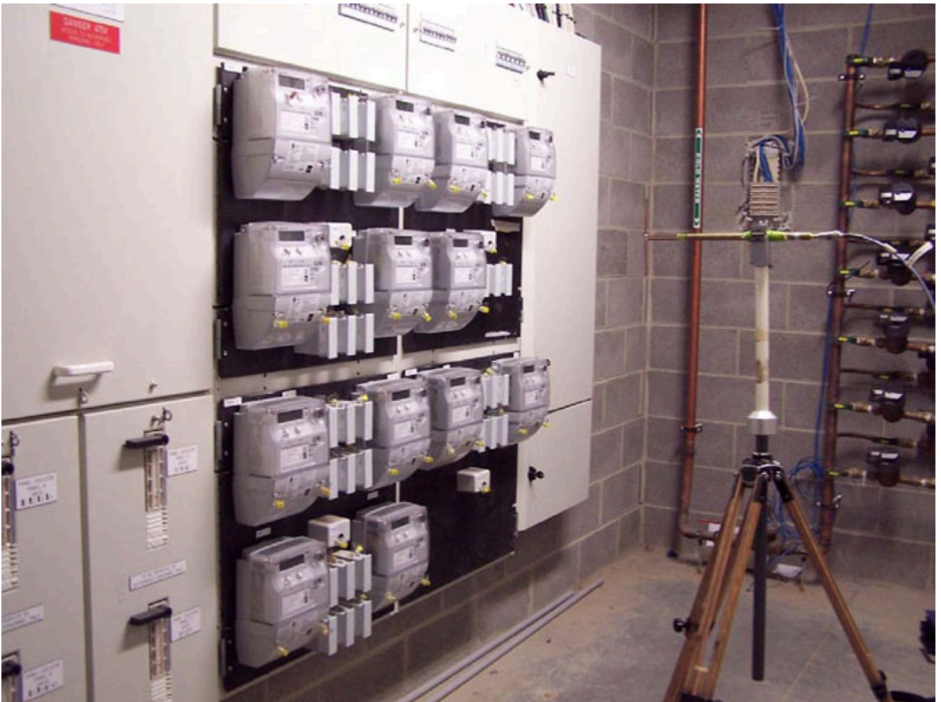
Figure 44 – Powercor Group Meter Site
